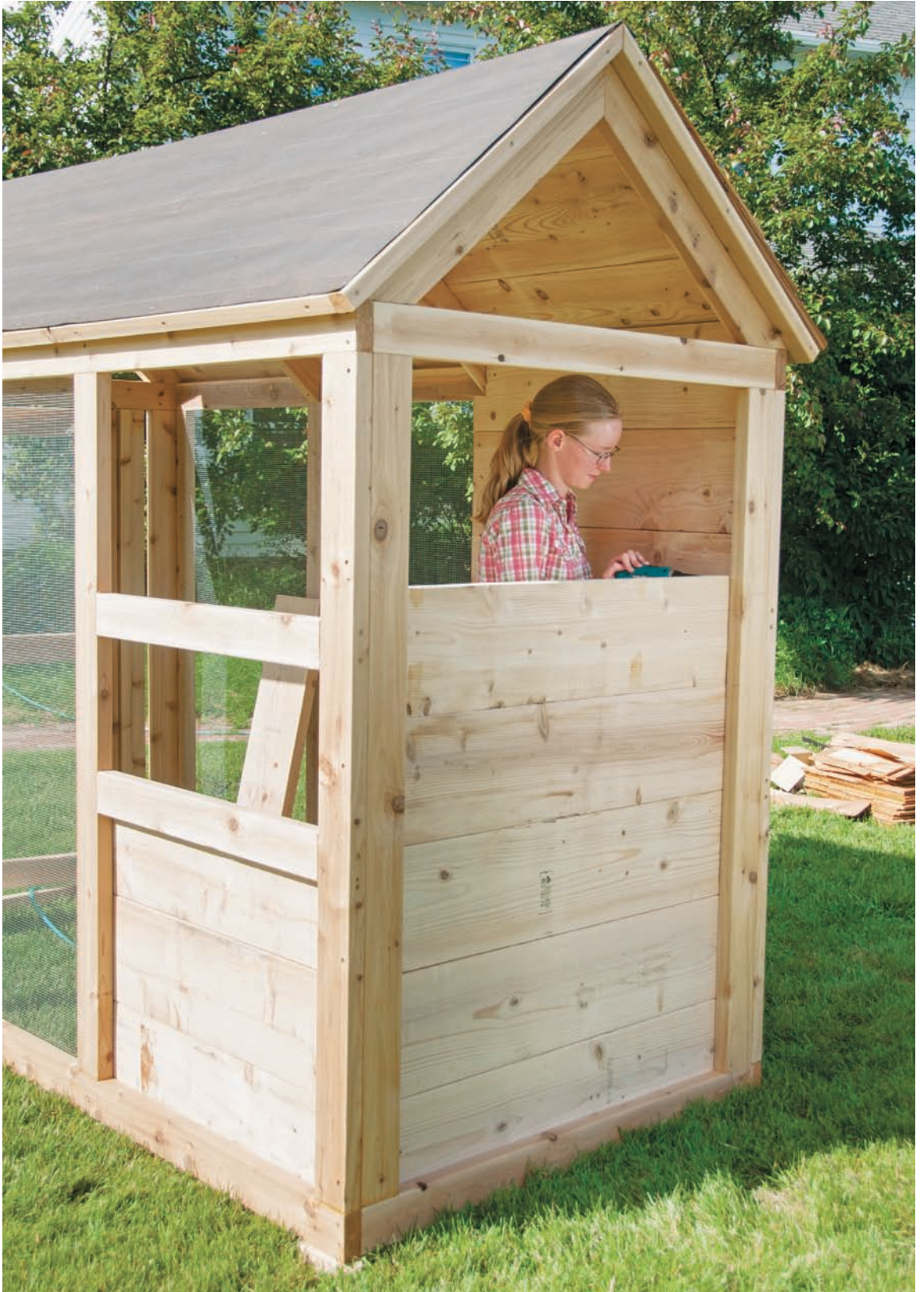
An in-process view of the construction of the back and side walls.
