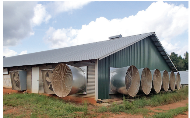
Figure 17.12 Large and smaller exhaust fans, respectively, moving air through a tunnel ventilation and side ventilation. (Photo courtesy of Michael Czarick, University of Georgia Cooperative Extension Service)
